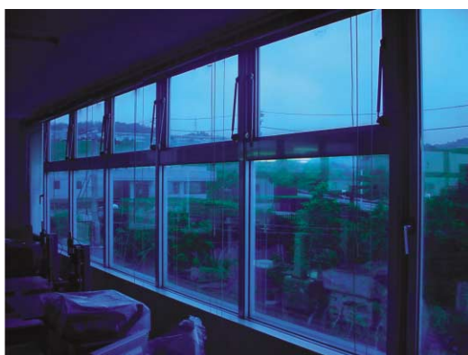
Thermal insulation film implemented on the inside of windows
