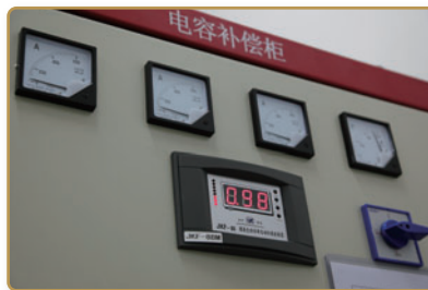
Equipment to increase power factor
