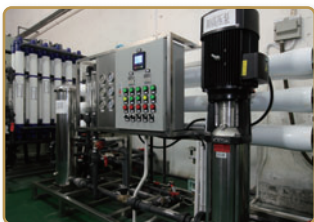
Equipment for reuse of electroplating wastewater
